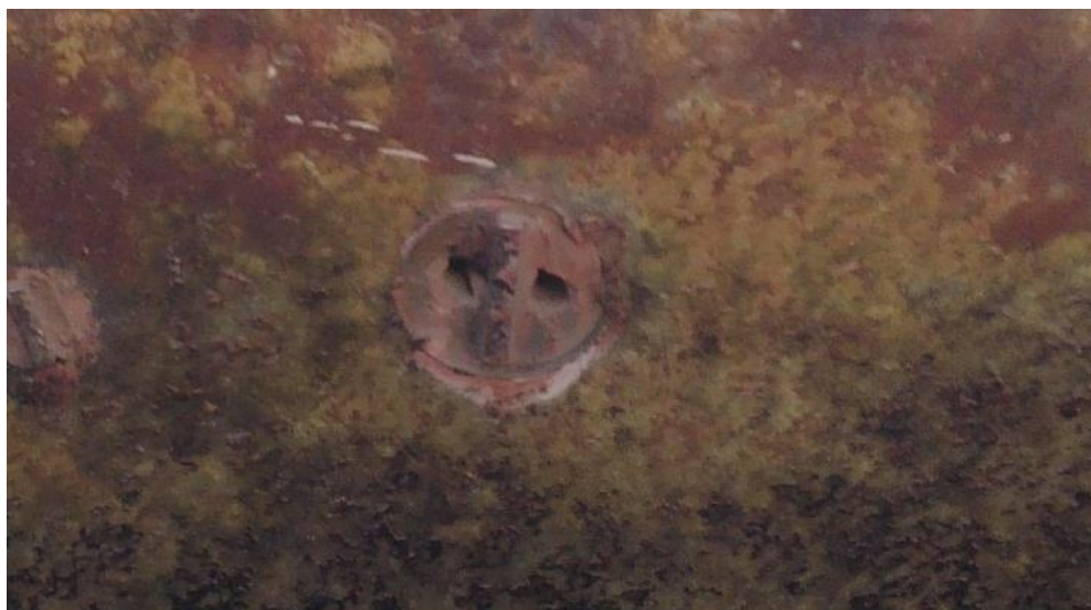
Measuring ports are open
