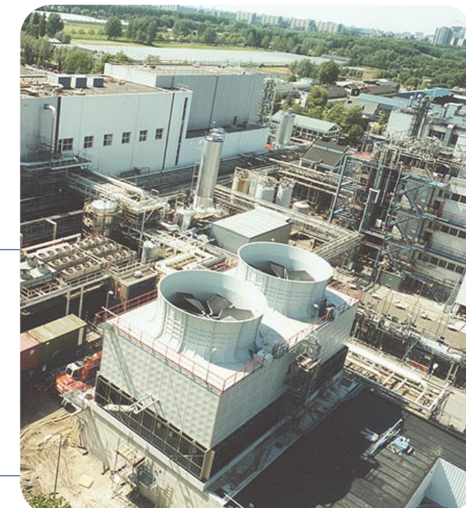
Left: SX fans in HVAC air-coolers. Right: ELFA fans in a cooling tower at a petro-chemical plant.
