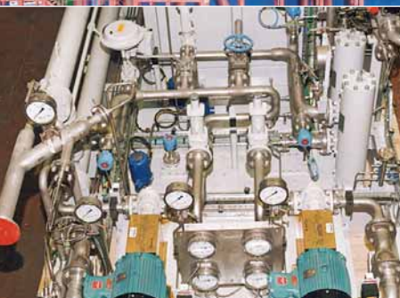
API614 lube system
