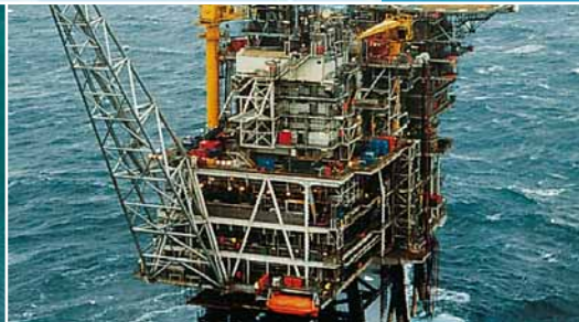
Fuel gas compression package for North Sea application. Courtesy of Chevron UK.
