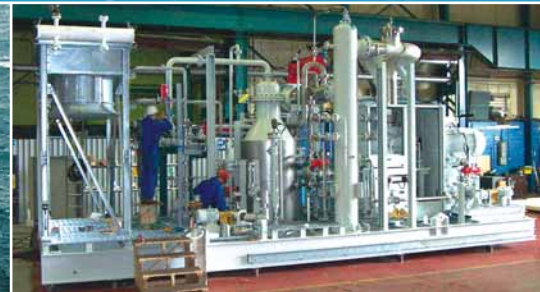
Flare gas recovery system for pilot plant in the Middle East.
