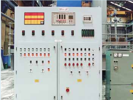
The compressor safe area panel for BP Amoco FPSO Schiehallion.
