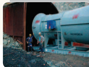
◀ Main Fan on Skid Mounts
