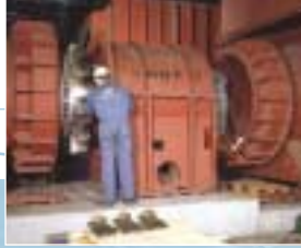
Rotating plant installation
