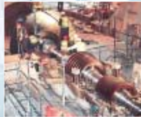
Rotating plant maintenance & servicing
