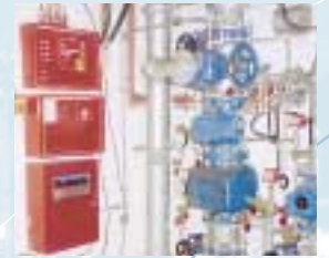
Fixed fire protection & detection systems: accredited to LPC standards
