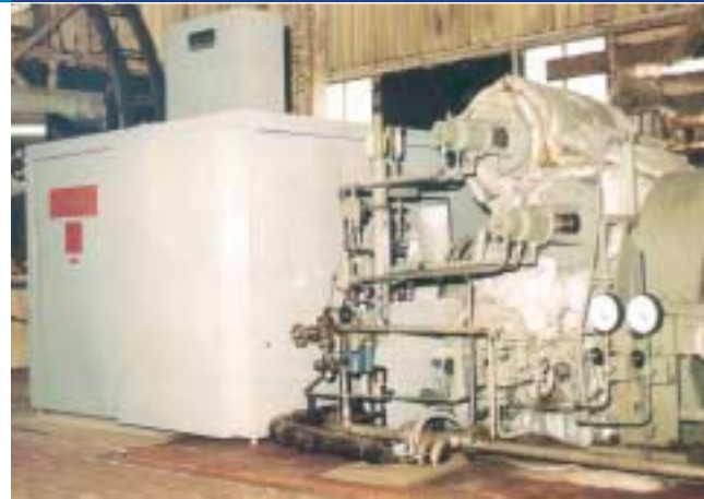
Howden installed steam turbine at a nitric acid plant
