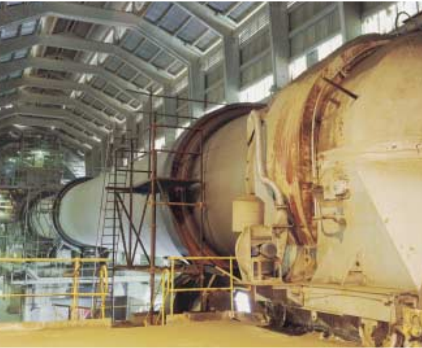
Refurbishment to cement kiln: replacement of splined tyre and 60 metres of drum
